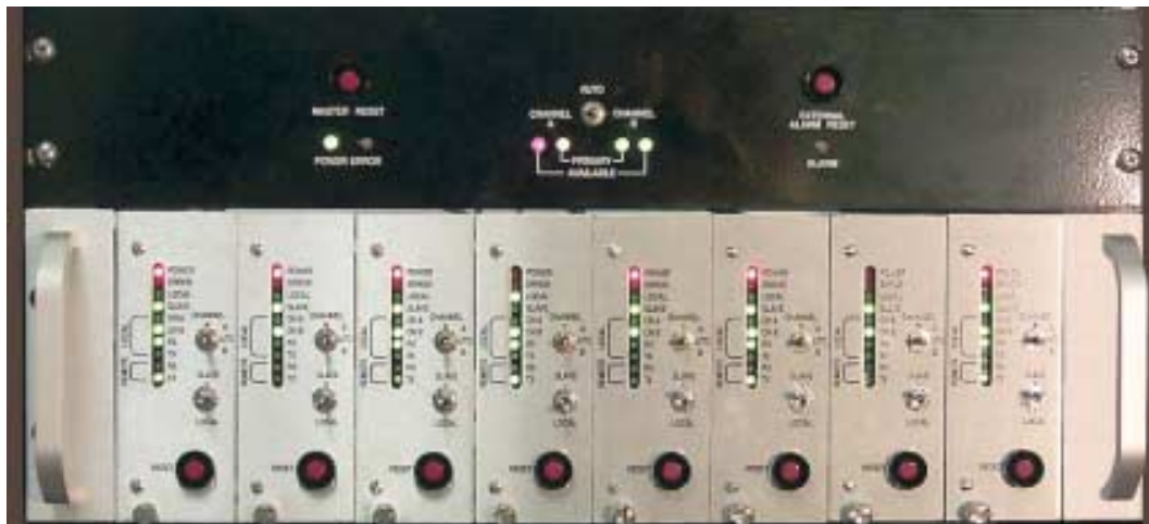
ATC rack-mounted controller and intelligent dual-ported serial interface switches
