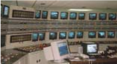
A tunnel control center at the Hampton Roads Bridge Tunnel
